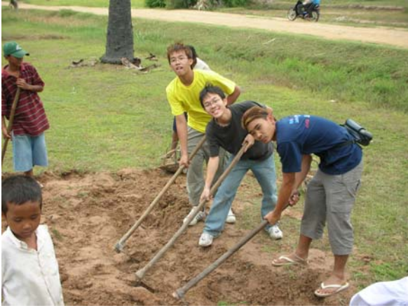
Z-Factor youths building a tar road as part of their overseas community service project at Cambodia
